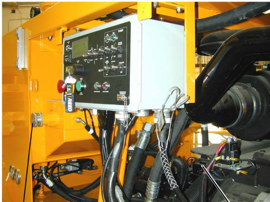
CONTROL BOX WITH COVER REMOVED
